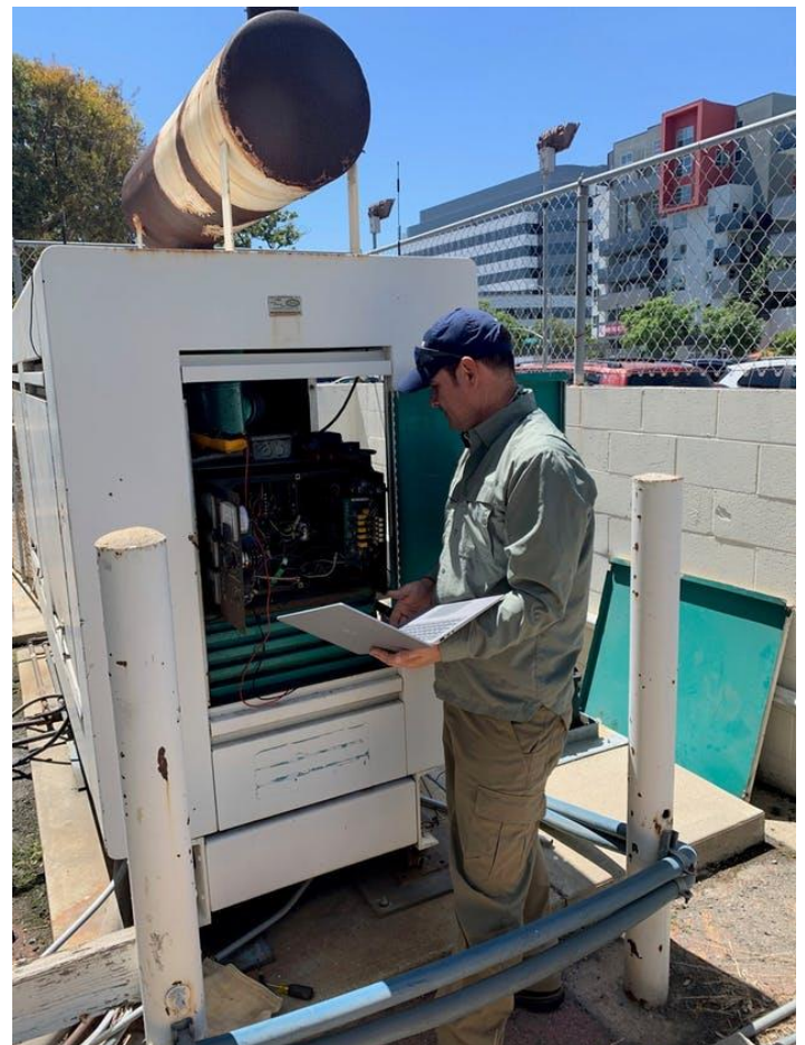
Tad Radecki, Chief of Installation Operations for PIONEER Systems, Inc., installs the first Power P.I.O.N.E.E.R. emergency power monitoring system at a Los Angeles County hospital on Aug. 4, 2021.
